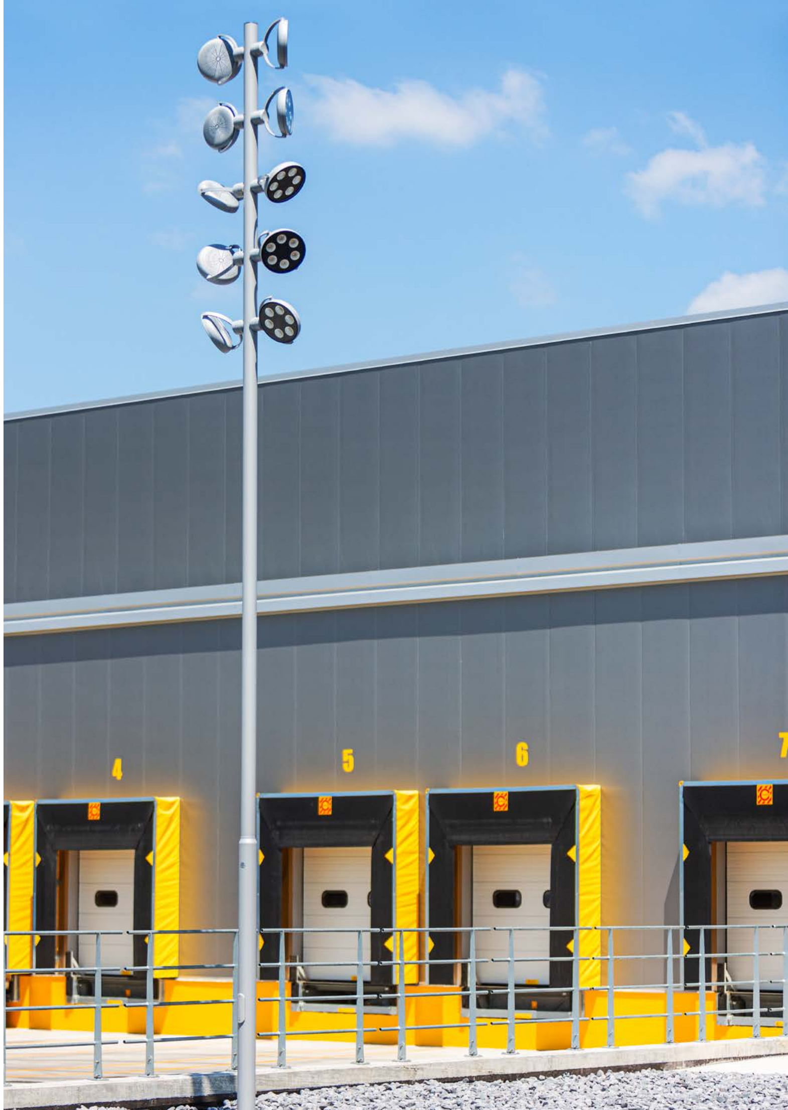
sun large floodlight on pole
