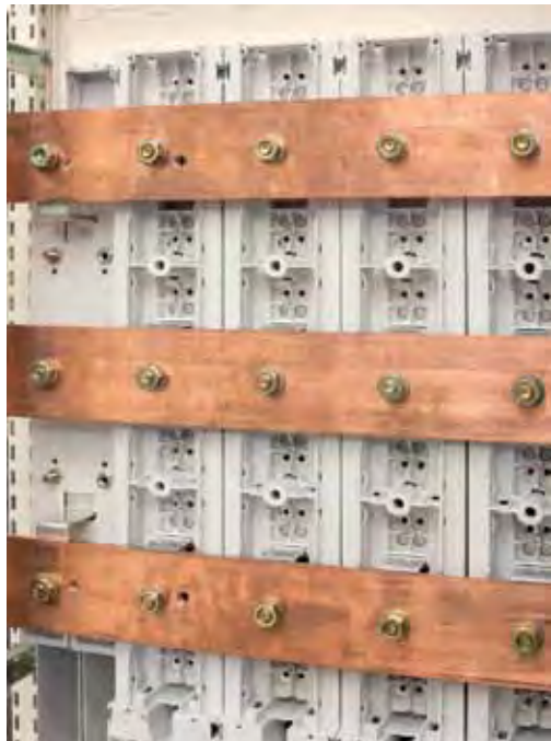
ISFL250 (direct connection on 185 mm² busbar).
